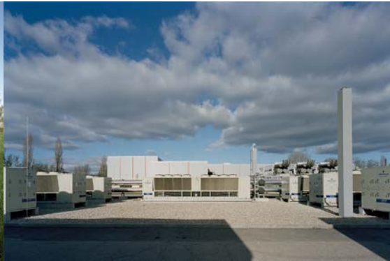
Datacenter in Berlin
