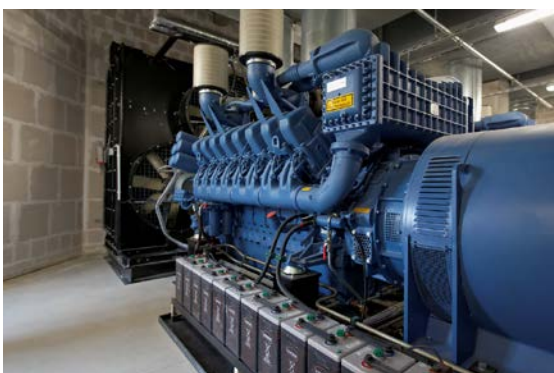
Generator facility of Datacenter in Frankfurt
