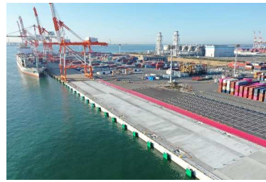
FY2020 Jetty superstructure work (No. 2) for east quay (-15m) of Tobishima pier in Nagoya port
